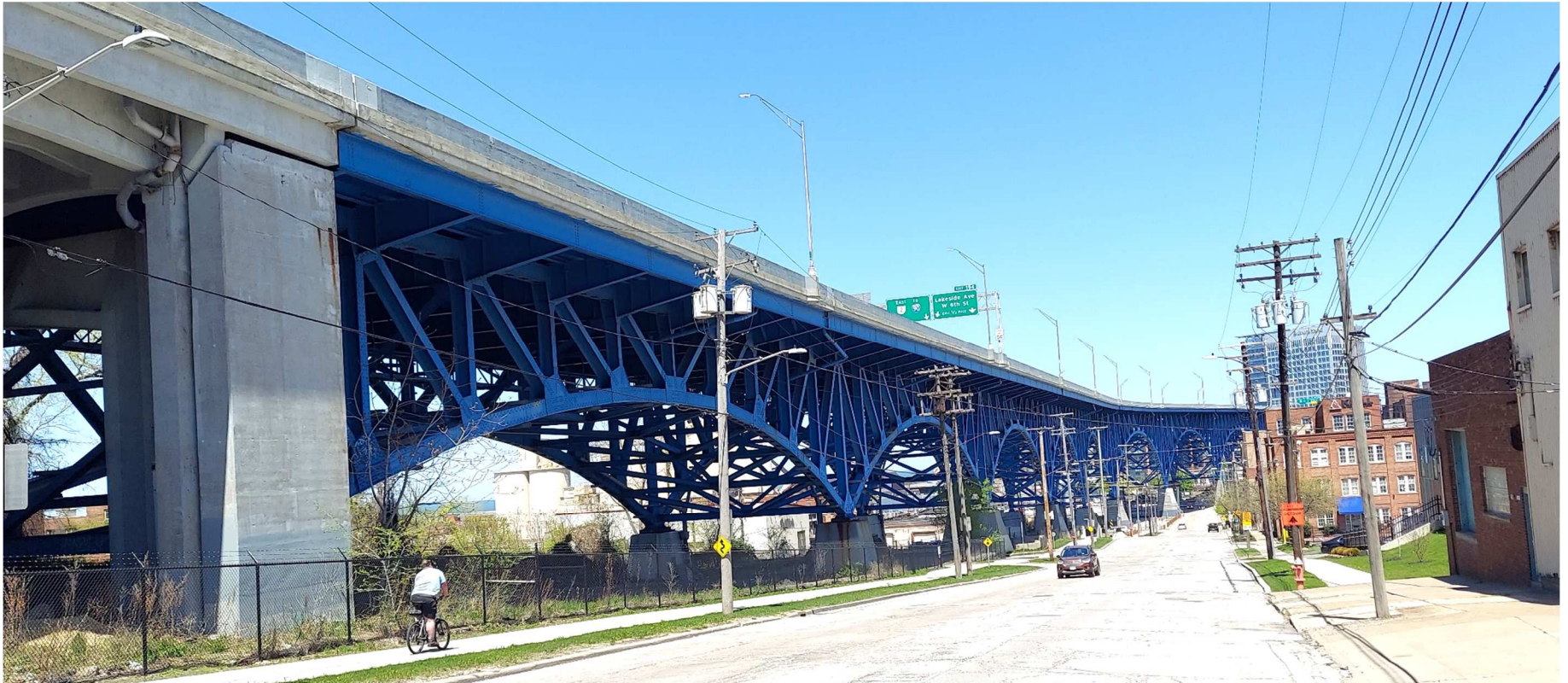
Figure 18: Beginning of main truss span is shown at left, where its replacement with a new bridge could begin per Concepts B-2, C-2, or D
